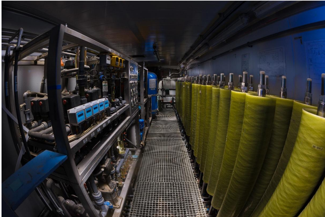
Inside a leachate treatment facility – RO-equipped mobile container by Klarwin
