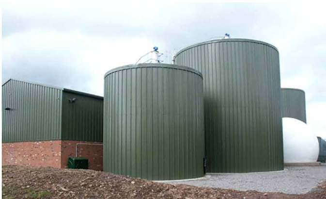
900 m 3 mesophilic digester, buffer tank, gas storage and digestate storage at the South Shropshire plant
