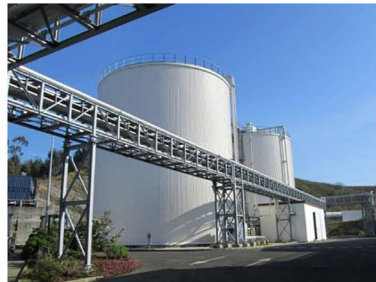
Two 3500 m 3 thermophilic digesters at the Valorsul AD plant in Lisbon
