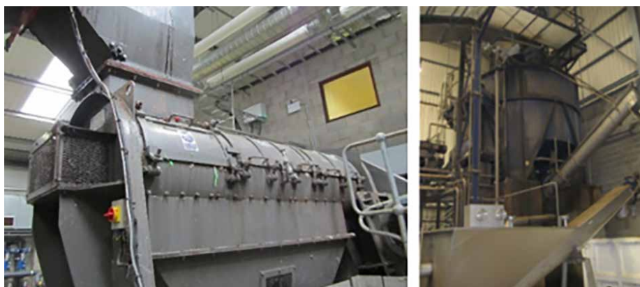
Figure 7: Left – Food de-packaging machine. Right – Linde hydropulper in operation at Valorsul AD plant (courtesy FP7 VALORGAS).
